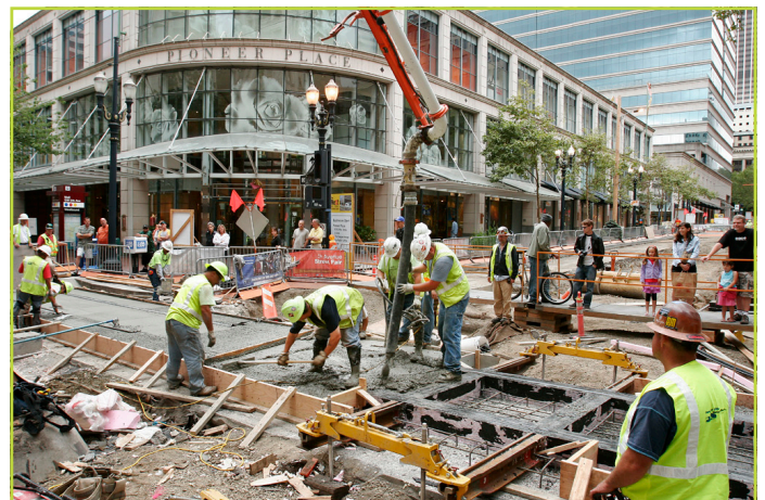
TriMet worked closely with contractors to speed construction. Crews worked double shifts in three to four block segments for up to eight weeks at a time.
